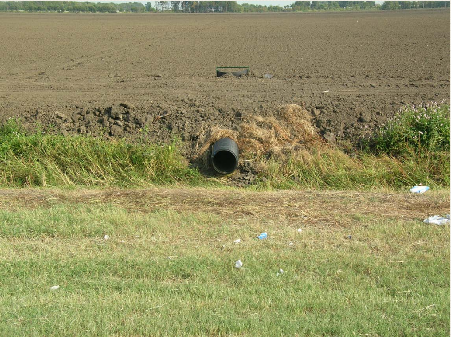
Pipe with water control structure
